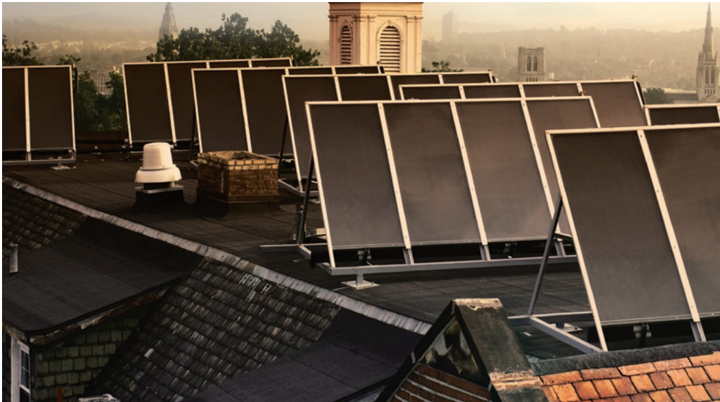
Solar thermal panels atop Woodland Hall
